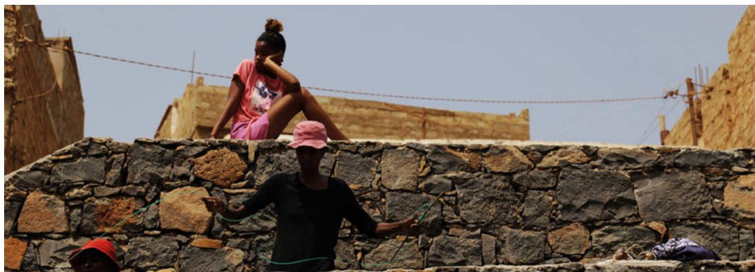
Moradora durante a obra do Alto de Bomba, Grace Ribeiro, 2021 / Resident during the construction of Alto de Bomba, Grace Ribeiro, 2021.
